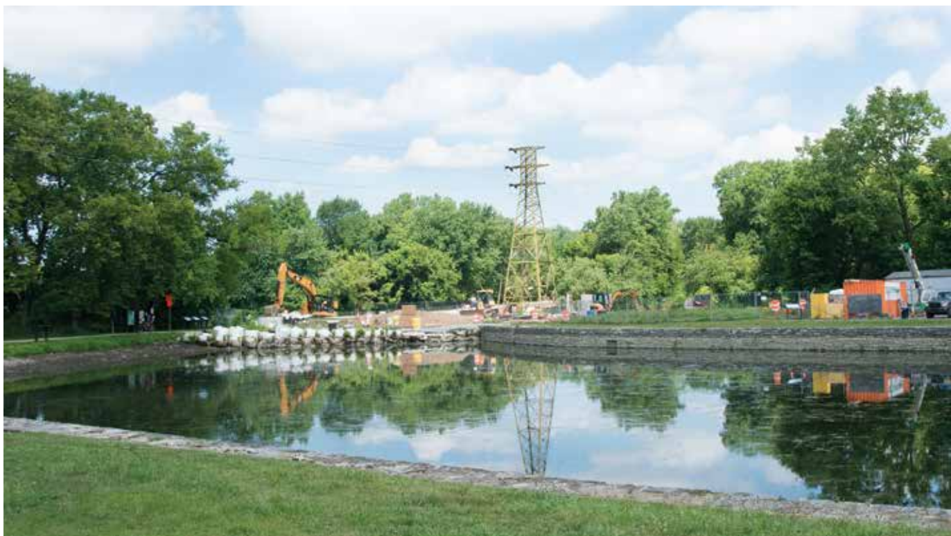
The Cushwa Basin was dammed to allow for the aqueduct restoration project.
