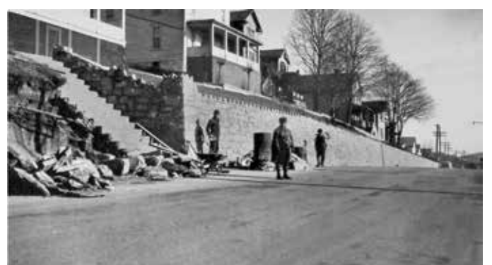
Top: The Frostburg Retaining Wall has stood the test of time for over 80 years.
