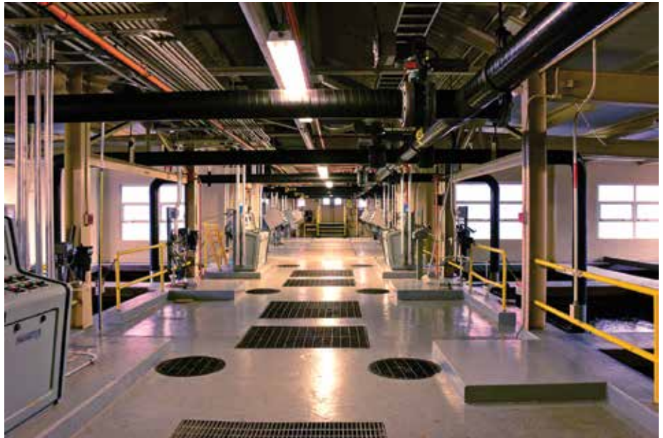
Inside a part of the Cumberland Filtration Plant — a sparkling clean facility.
